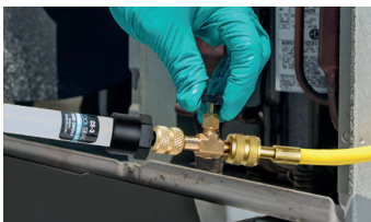
Charge inline with refrigerant
